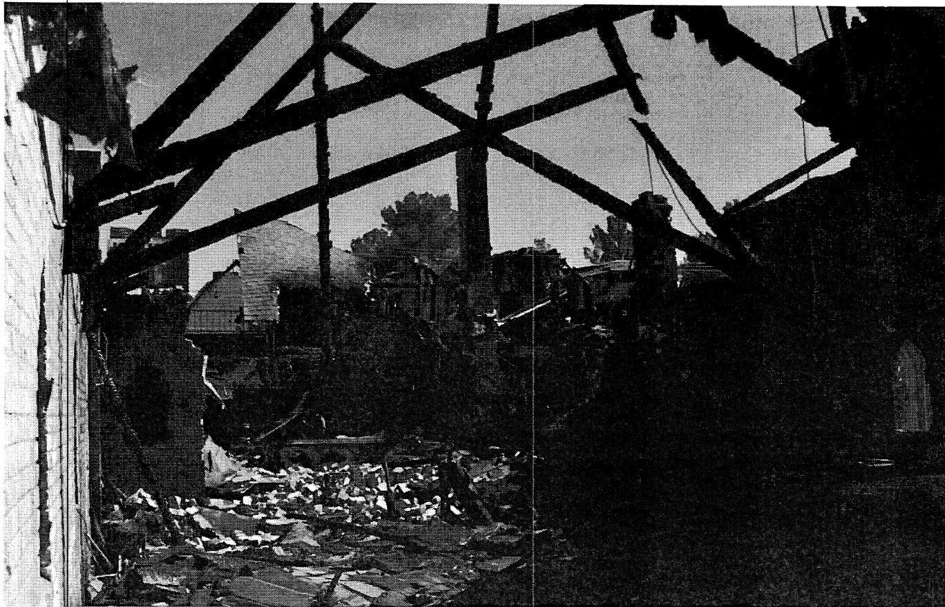
Fire damage at Saint Stephen's Episcopal Church building
