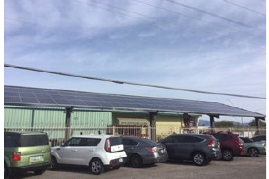
Exterior of Sister Jose Women's center with solar panels installed using CDBG dollars.
